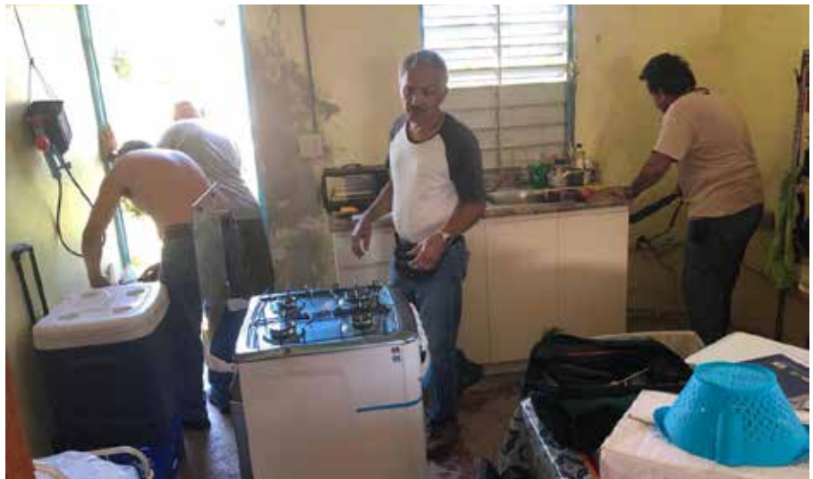
MIMITA NIEVES (ABOVE) SHOWING PRESBYTERIAN VOLUNTEER THE DAMAGE TO HER HOME. THE VOLUNTEERS HELPED HER CLEAN AND MAKE NECESSARY REPAIRS. PHOTOS: PRESBYTERIAN NEWS SERVICE
